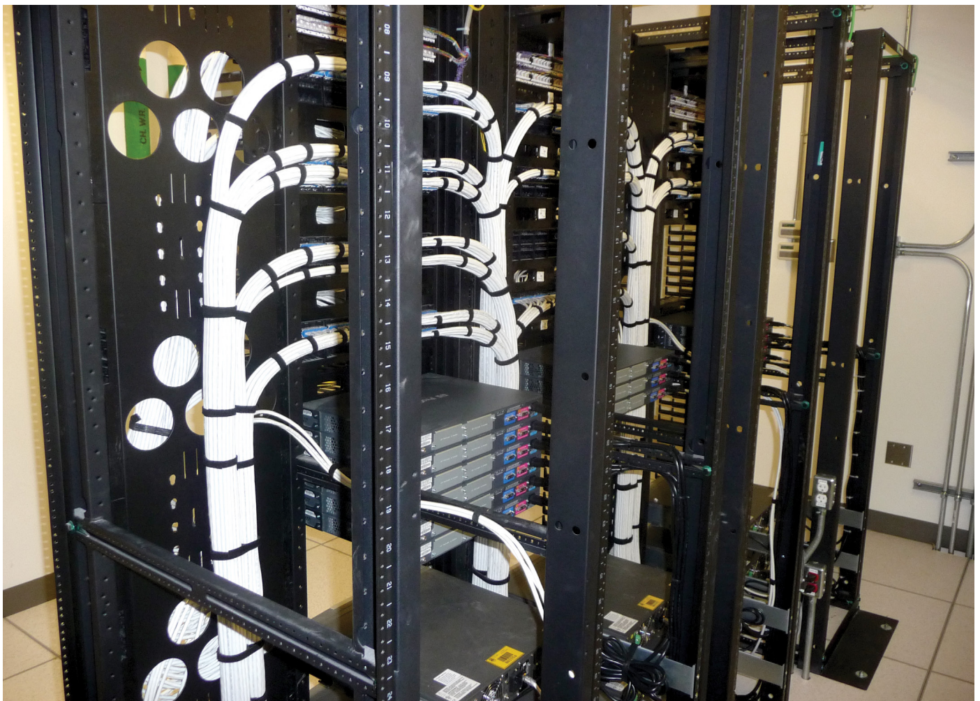
FIGURE 3: Managing category 6A at the rack.
